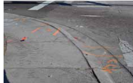
Non ADA compliant pedestrian curb ramp
