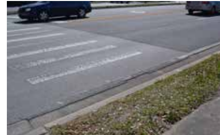
Lack of pedestrian curb ramp at Casselberry Commons entrance
