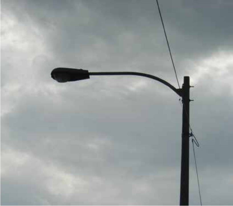
Figure 1 Street lights used on Colonial Drive
