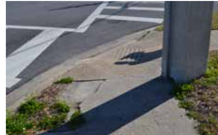
Non ADA compliant pedestrian curb ramp
