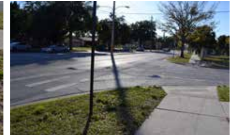
No directional curb ramps and faded markings
