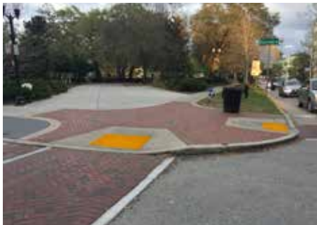
ADA Pedestrian Directional Ramps Photo Credit: KAI
