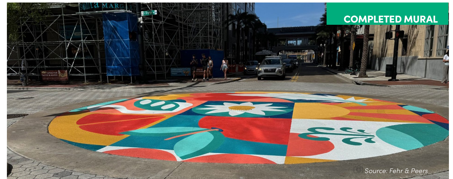
Construction in action of an intersection mural in Downtown Orlando (Intersection of Orange Avenue at Church Street) as part of a Quick Build project.
